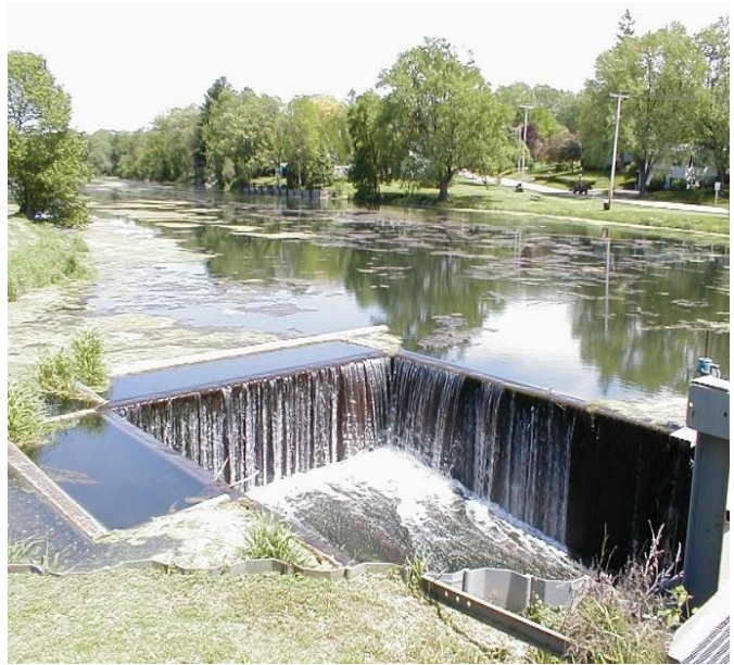
Dense aquatic plant growth in an impounded river with a water level control structure
