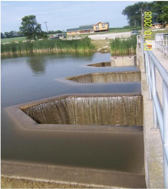
The dam and outflow structure determine how much water levels can be lowered
